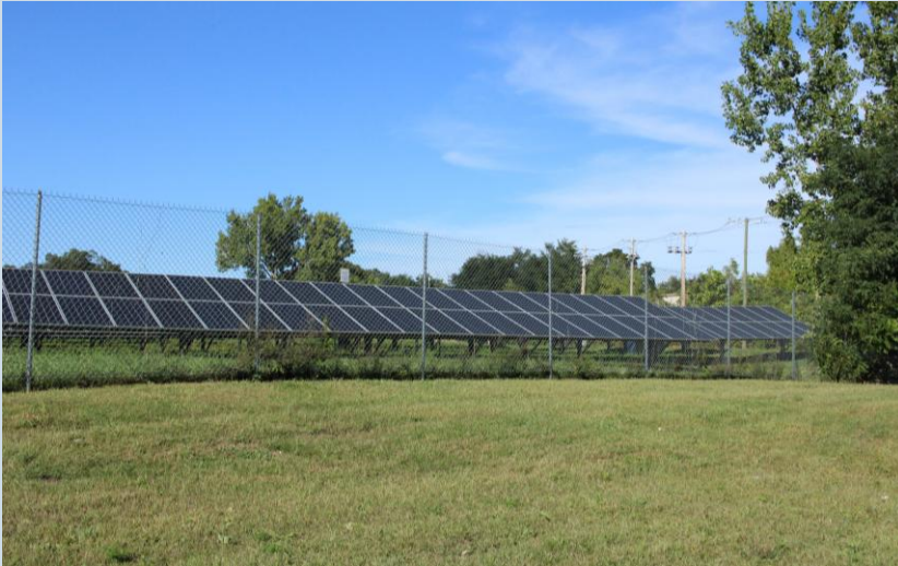
Solar Facility on Oak Street
