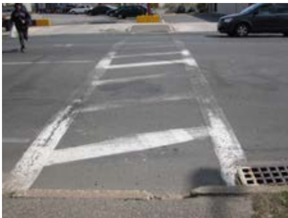
Non ADA compliant pedestrian crossing
