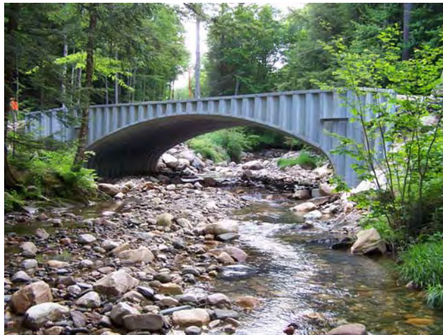
Dingle Road crossing of Bronson Brook, Worthington, after. (Credit: Carrie Banks)
