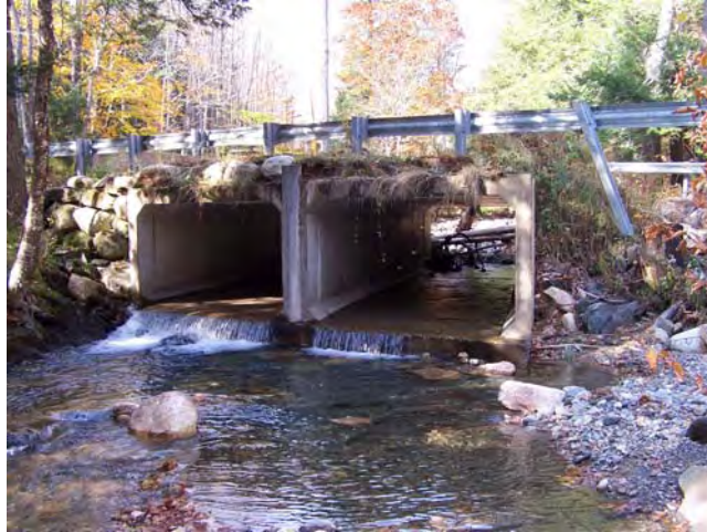
Dingle Road crossing of Bronson Brook, Worthington, before. (Credit: Carrie Banks)
